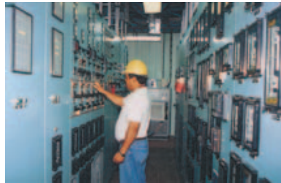
ETESA At work in the control room of the new Panama II sub-station.
