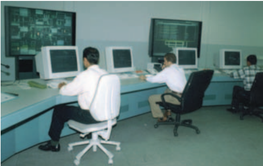
GECOL is responsible for generation, transmission, and distribution of electric power throughout Libya.
