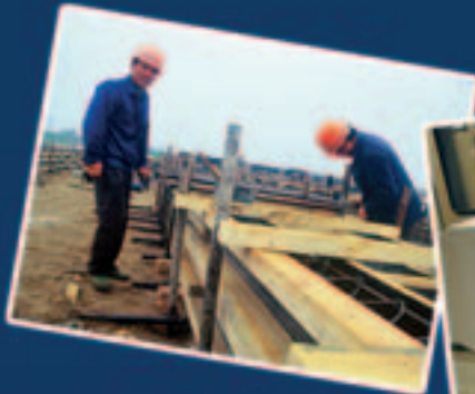
Henan Kaifeng Carbon Manufacturing Plant, China
