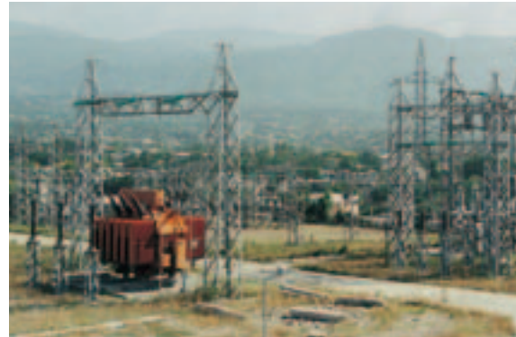
POWERING THE LAND The government is exploring the possibility of using alternative energy sources such as water.
