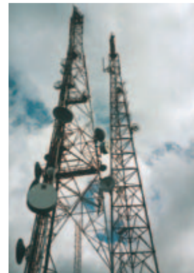
CONNECTING HAITI TO THE WORLD The recently liberalized Haitian telecommunications sector is to be regulated by Conatel.
